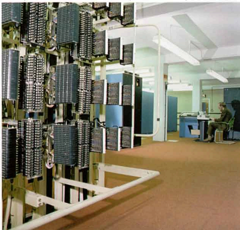
The telephone equipment room at Atlantic House housing the IBM 3750
