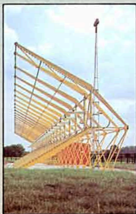
Side view of ILS localiser aerial
