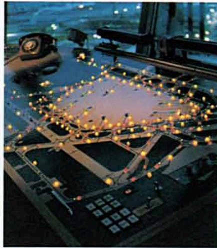
The airfield lighting control panel
