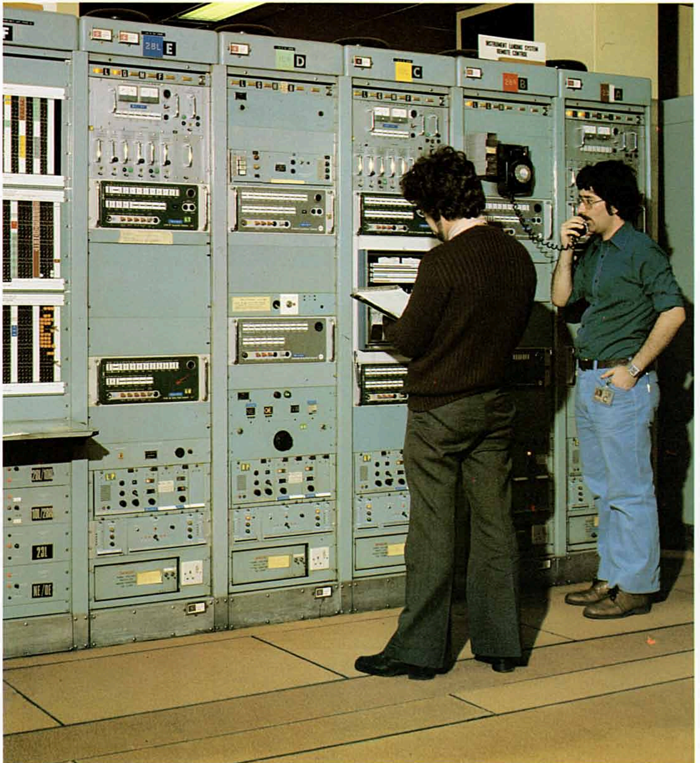
Below Instrument landing system monitoring bay in the Telecommunications Equipment Room
