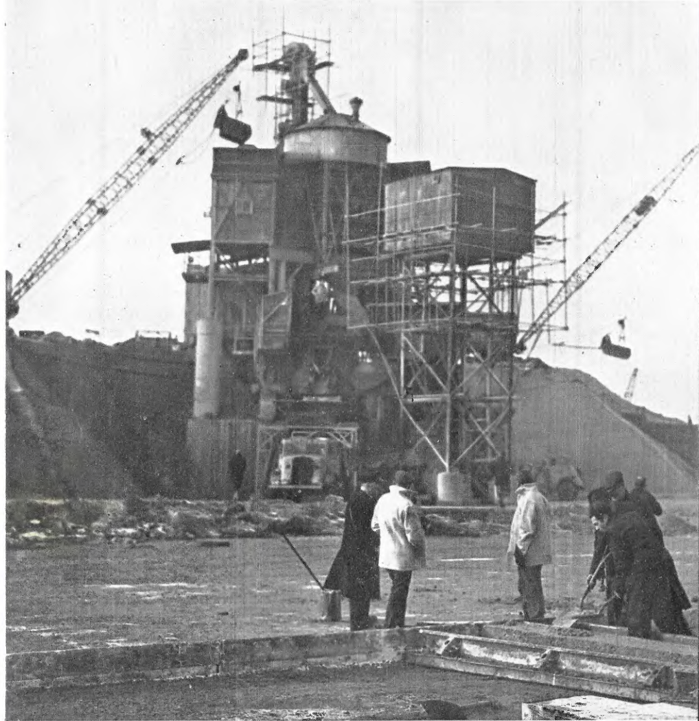
The concrete-mixer in the background is one of the world's largest. In the foreground, a new runway takes shape.
