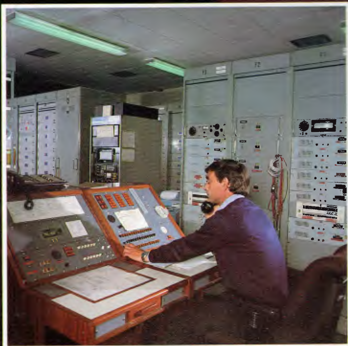
The Telecommunications equipment room
